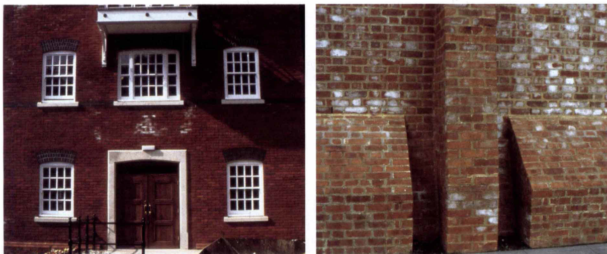
Figure 3 Efflorescence (salt deposits) showing up as white patches on a house and a wall (Pictures reproduced by courtesy of the Brick Development Association www.brick.org.uk )
