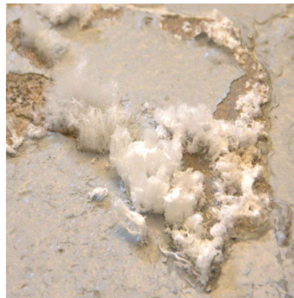
Primary efflorescence showing the appearance of salt crystals emanating from concrete
