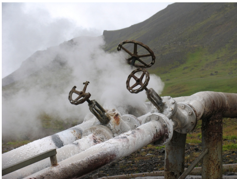
Figure 2: Formation of limescale deposit around leaking valves
